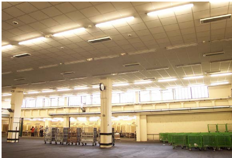
With radiant heaters, the heat is transferred to surfaces such as people, floors and fixtures. This creates comfort even in rooms with large volume.
